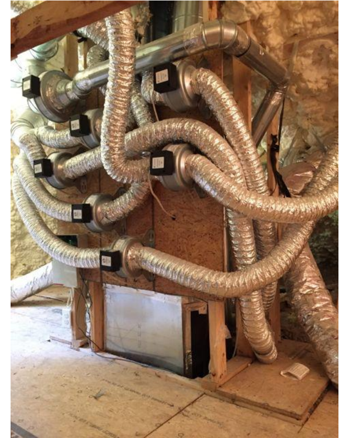
Single family home bath fan ducts Photo: Energy Vanguard
