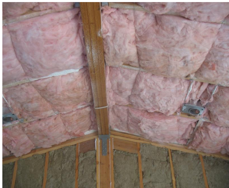
Remaining cavity is filled with Batt Insulation. (Blown-in insulation would also be acceptable.)
