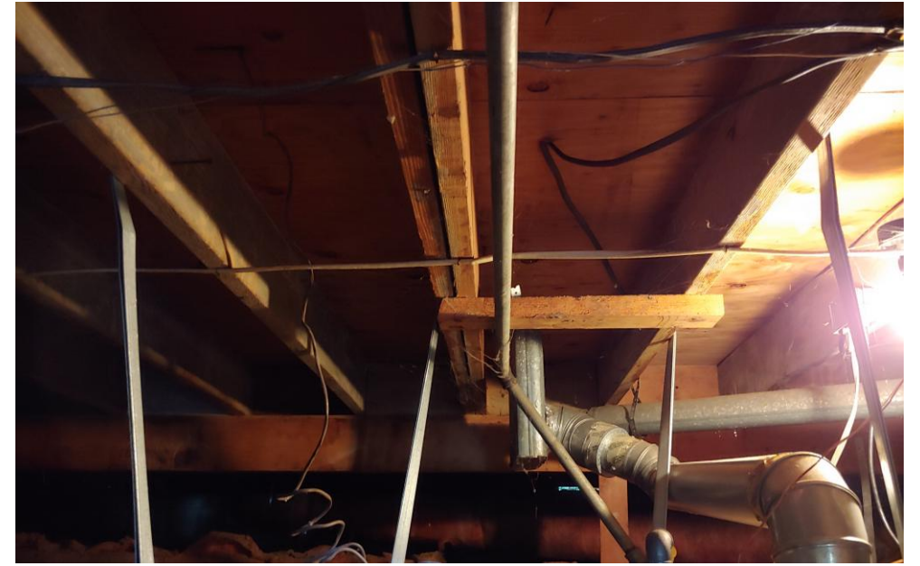
Existing Raised Floor without Insulation nor Air-Sealing
