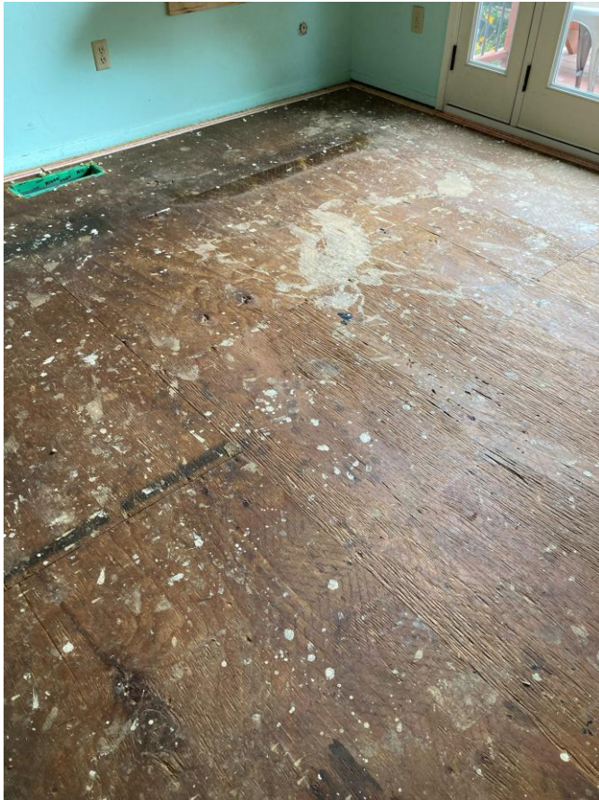
Existing Floor was not an Effective Air-Barrier
