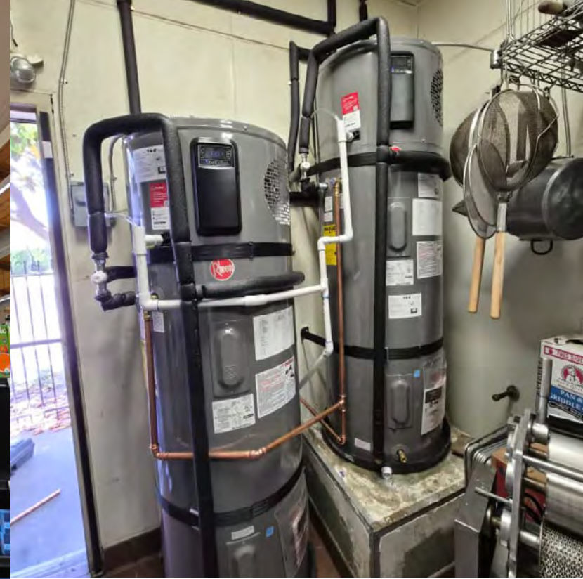
Heat pump water heaters provide hot water to a taqueria in Santa Maria.
