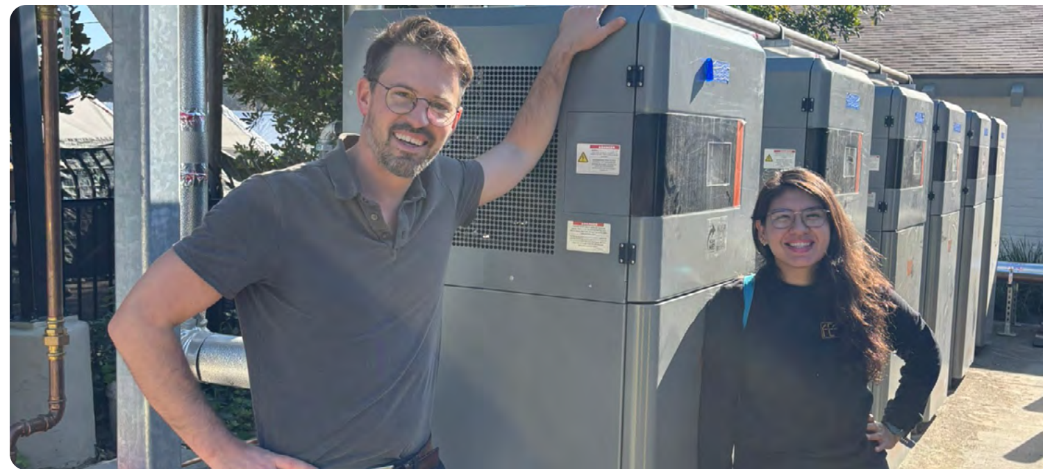
America Diaz (3C-REN Technical Assistant) and David Ross (Senior Project Manager from Ventura Housing, the housing authority of the City of Ventura) in front of Valentine Road Apartment's central heat pump water heating system.
