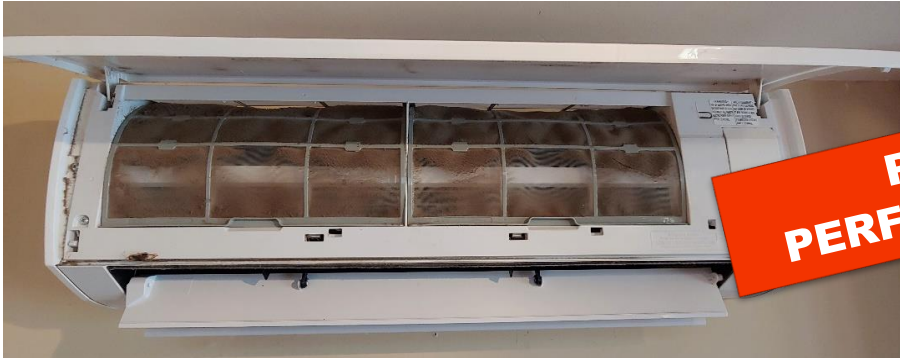
Under the Hood –with dirty Filters
