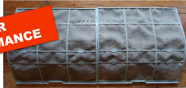
Dirt and Dust Build-up
